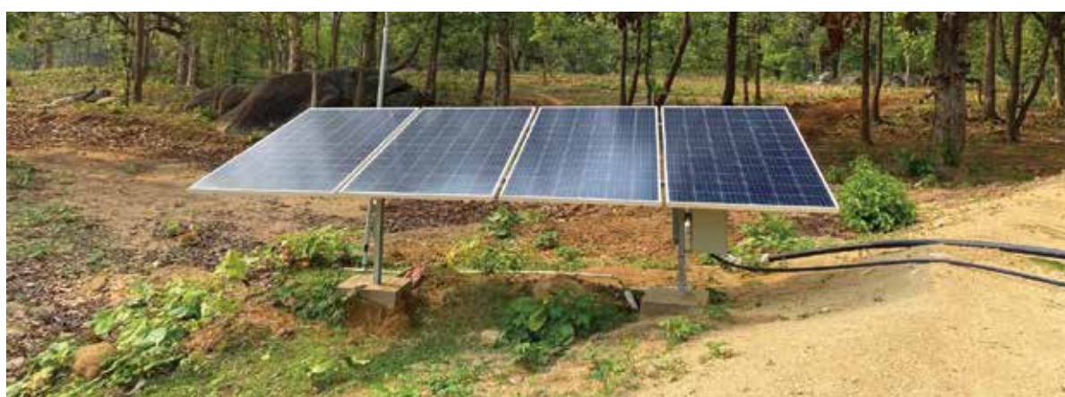
Solar Water Pump
