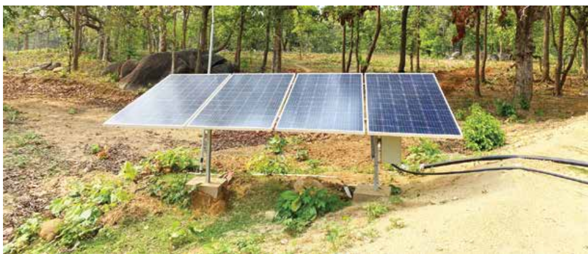
Installed Solar Water Pump in Community
